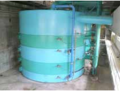
Downstream sand filter
